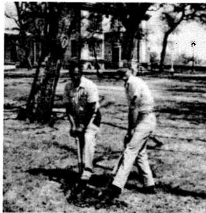
Left: Isaac Harper, Grounds Maintenance Leader & Stephen Schoen, Groundskeeper repairing sprinkler heads at Little Campus
